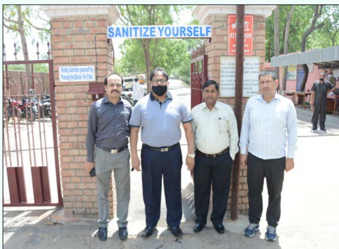
Installation of Sanitizer Pass Way at Main Gate of BRCM Vidyagram Campus
